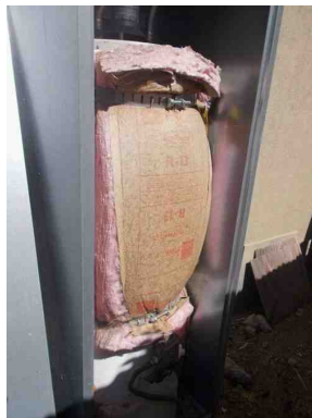
Water Heater - 2 Straps
