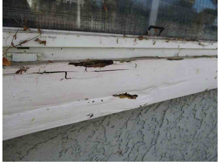
Peeling Paint/Wood Rot
