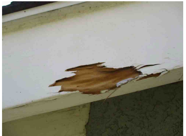
Termite Damage to Eaves
