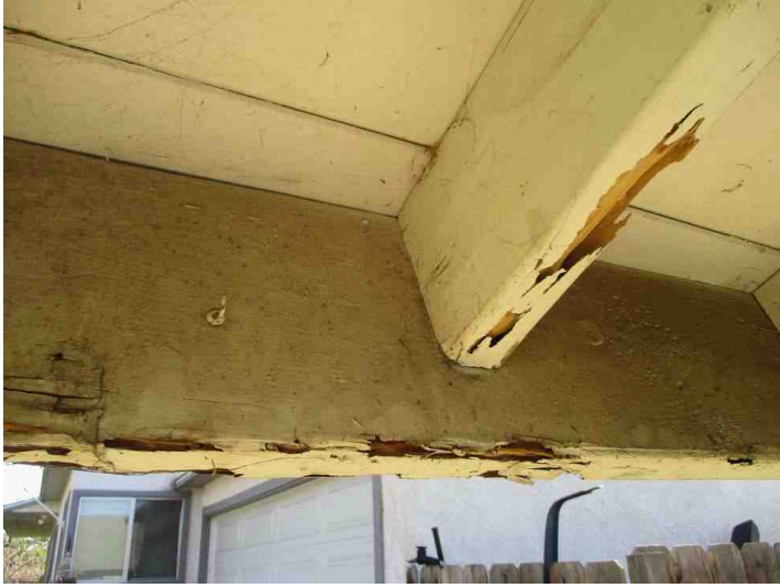
Termite Damage on Eaves/Peeling Paint/Wood Rot
