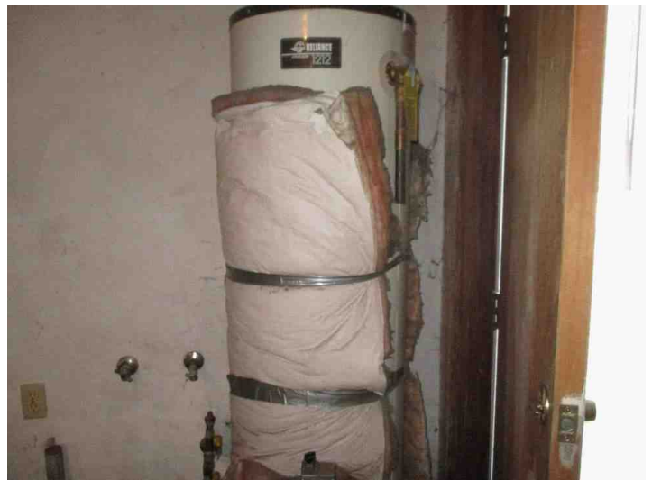
Water Heater (Strapped)
