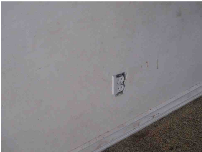
Broken Outlet Covers
